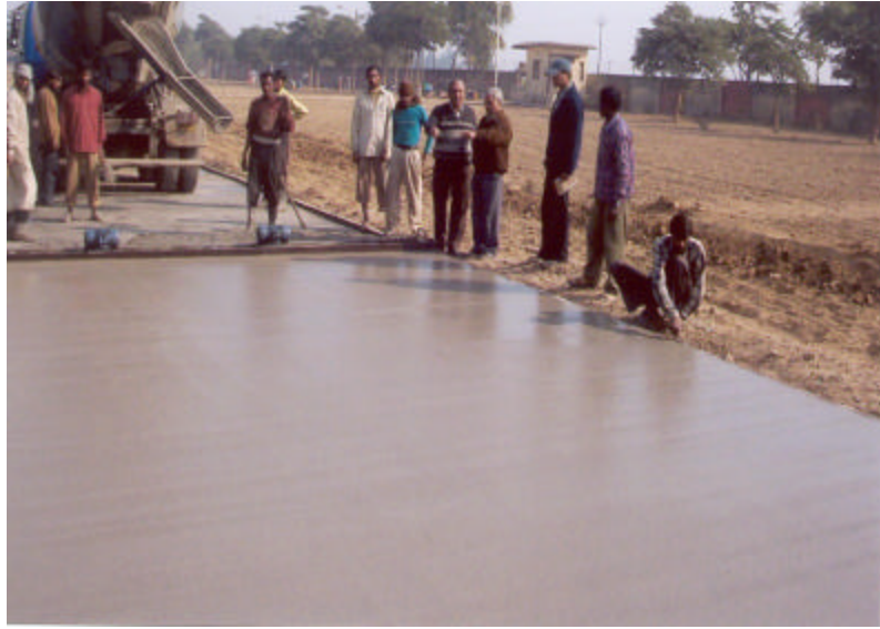
Fig.2: Laying of Ultra Thin White Topping (50 mm Thick) at HRDC Centre of CSIR at Ghaziabad
