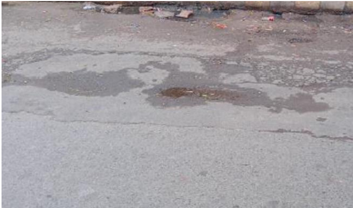
Figure 11: Cracking observed on the study road
