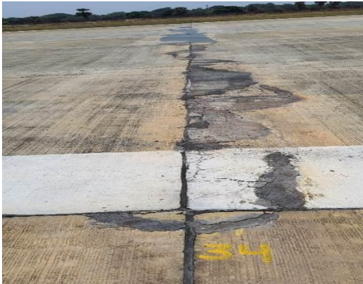
Figure 8: Deteriorated condition of the repaired expansion joint
