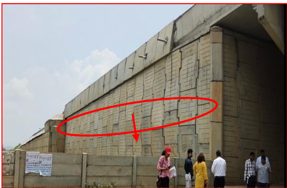
Figure 4:(b) Bulging of panels (RHS)
