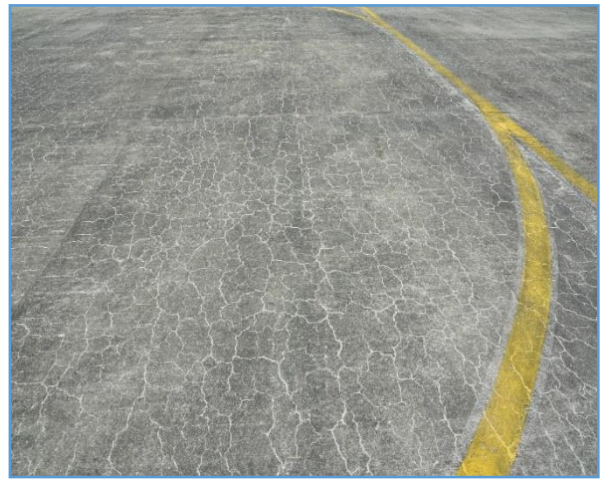
Longitudinal Cracks on
