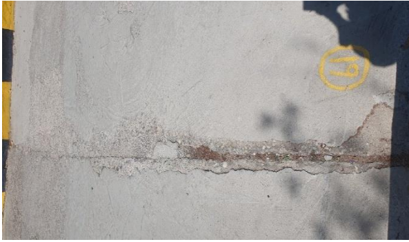
Fig 13: Severely deteriorated spalled transverse joint
