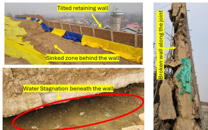
Figure 1: Images of the failed retaining wall along the AB section
