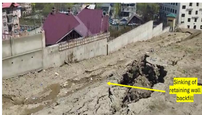
Figure 2: Failed retaining wall at the KL section
