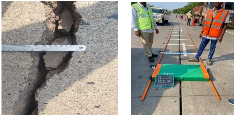
Fig. 2: Single longitudinal crack of 90 mm & MIT scan test under process
