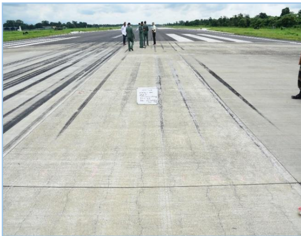
Slab showing Alligator pavement Slab at Runway
