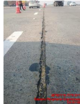
Photo 23: Lane Separation between Lane L4 and L5, width of 15-20mm
