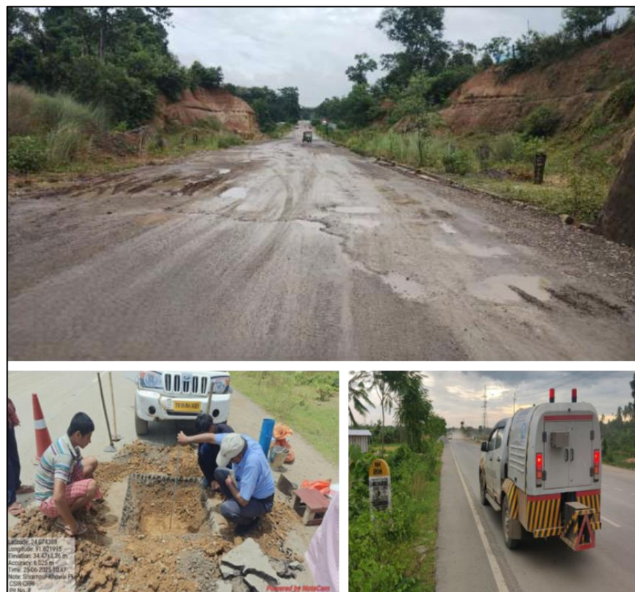
Photo 14: Distressed pavement and site investigations
