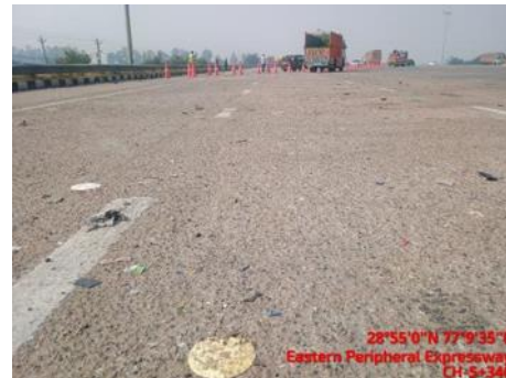
Photo 25: A view of the Surface scaling observed on the concrete pavement
