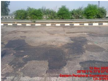
Photo 24: Settlement observed on full carriageway repaired with bituminous carpet
