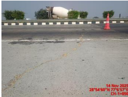
Photo 22: Diagonal Crack on full carriageway with spalling over the crack
