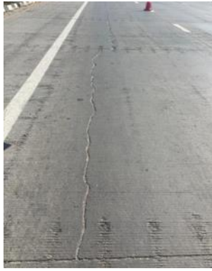
Photo 20: Longitudinal Crack in L3 at CH 19.800
