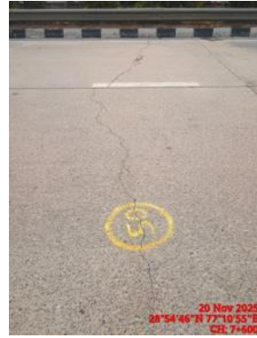
Photo 21: Transverse Crack in Lanes L1 to L3 at the middle of the panel
