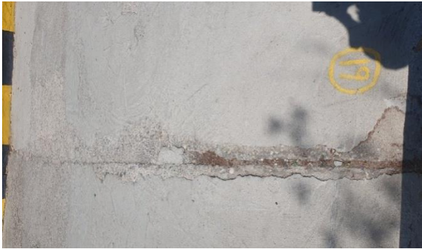
Photo 32: Severely deteriorated spalled transverse joint
