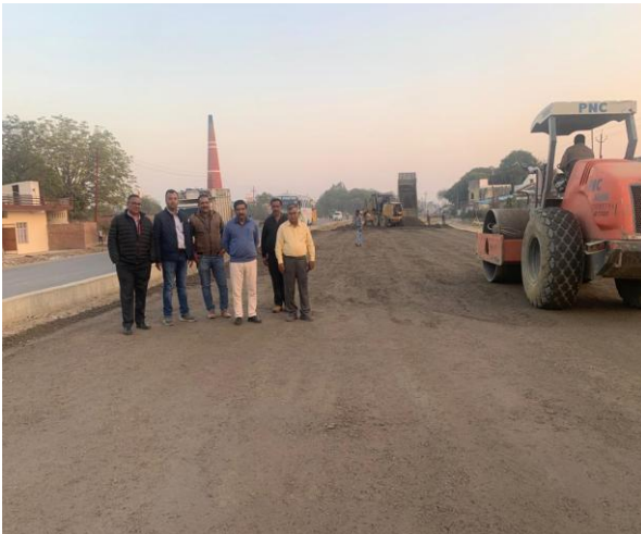
Figure 1(a): Laying and Compaction of the Stabilized Sub-Base Layer in Uttar Pradesh
