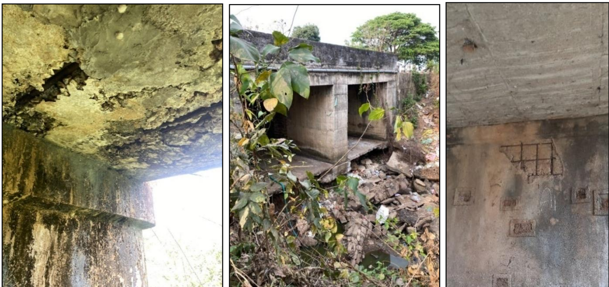
Figure 16: A Typical View of (a) Severely Exposed Reinforcement Observed on the Deck Slab of the Paiki Nallha Minor Bridge on Bhanjanagar- Tillisingi -Tarasingi Road at Ch. 29.550. (b) Erosion of the Apron of the Kotibaradi Bada Sankh Nallha Bridge on Bhanjanagar Tillisingi Tarasingi Daspalla Road at Ch. 9.580 Km in Bhanjanagar Division (c) Exposed Reinforcement on the Abutment of the Sulia Bridge in Nayagarh-Odagaon-Laukhala Road at Ch. 4.770 in Nayagarh(R&B) Division.
