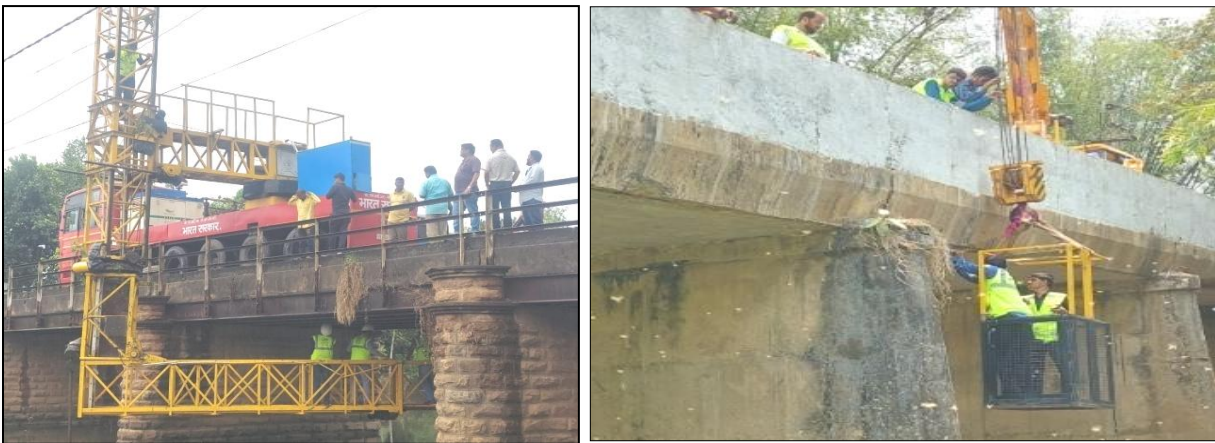
Figure 15: A Typical View of (a) Inspection of Superstructures of HL Bridge over Dhanei River in Budhamba-Buguda road at Chainage 8.988 Km in the Bhananagar Division using MBIU. (b) NDT on the Deck Slab of the Bridge over Local Nalla on Koilama-Brundabanpur Road at Ch-6.200 in Nayagarh(R&B) Division.
