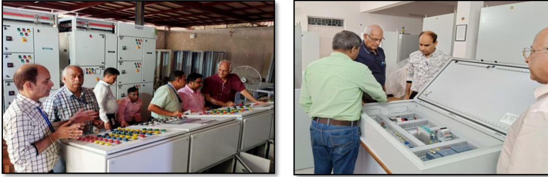
Figure 12: Showing PDI of PKG2 Electrical Panels and PDI of PKG-3 Control Panels
