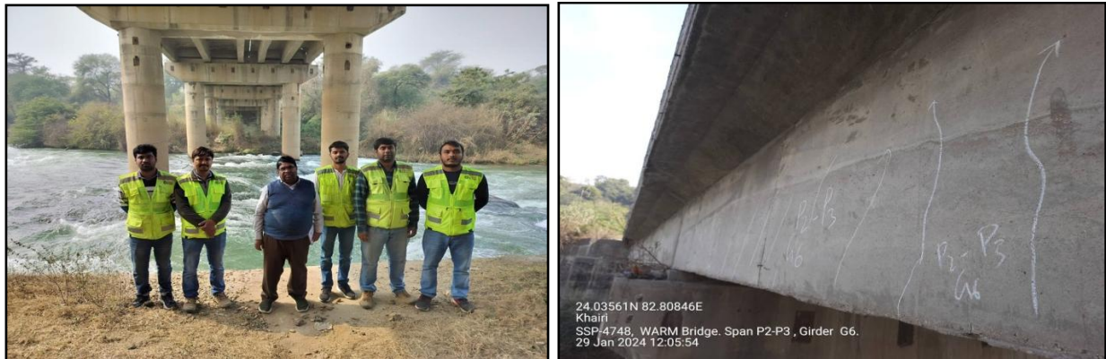
Figure 24: A Typical View of (a) Inspection and (b) Cracks Observed on Girder G-6 In Span P2-P3 of Warm Bridge of the NTPC at Rihand.
