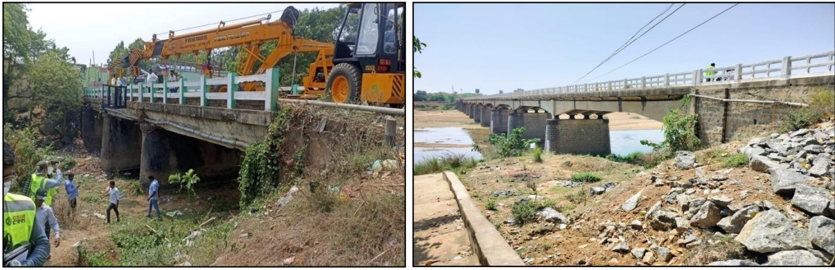
Figure 14: Inspection of (a) Sulia Bridge using a Man lifter on Nayagarh-Odagaon-Laukhala Road at Ch. 4.770 in Nayagarh(R&B) Division. (b) Rushikulya Bridge in Purushottampur-Jagannathpur Road at Chainage 2.700 Km in the Ganjam-II Division.
