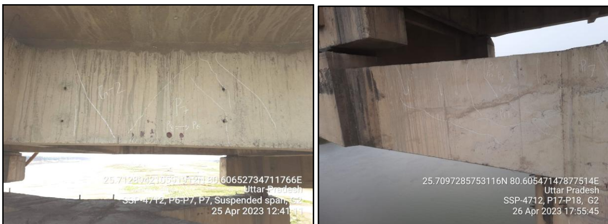
Figure 19: A Typical View of the Crack Observed on Girder G2 in the Suspended Gap Span at Pier P-7 of Yamuna Bridge at Bendaghat. (b) Severe Cracks observed on Cantilever Supporting Bracket below Girder G-2(RHS) at Pier Head of Pier P17 in the Span P17-P18 of Yamuna Bridge at Bendaghat.
