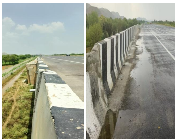
Figure 5:(a) Tilting of MSE wall crash barrier towards the road surface
