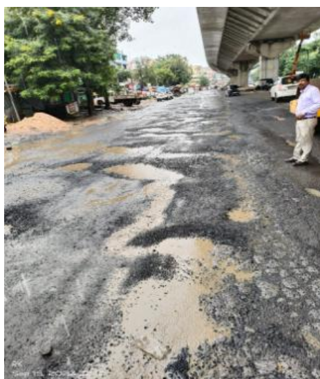
Figure 3: A typical photo showing the existing condition of the pavement
