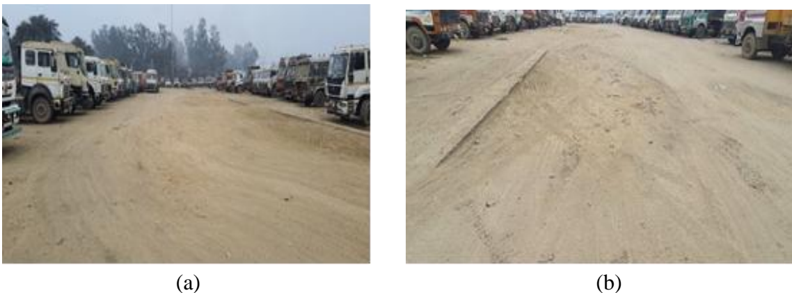
Figure 7: (a) A view of the existing distressed truck parking area used by Multi axle container trucks, (b) A view of the large potholes developed in the existing pavement
