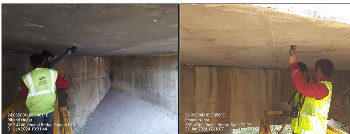
Figure 26: A Typical View of Non-Destructive Testing of the Deck Slab of Span A1-P1 and P2-P3 of Chahal Bridge of the NTPC at Rihand.
