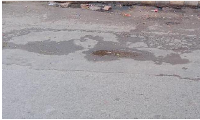
Figure 11: Cracking observed on the study road
