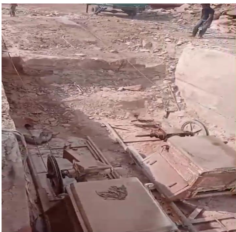
Figure 3: Recommended Diamond Rock Cutting method for the protection of Chandpur-Jhansi ancient monuments from vibration
