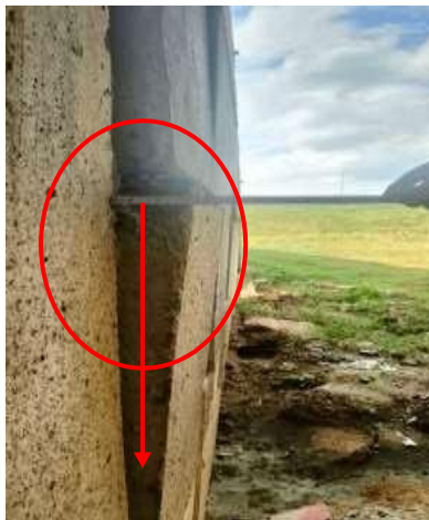
Figure 3: Panel dislocated from the joints at in the corner
