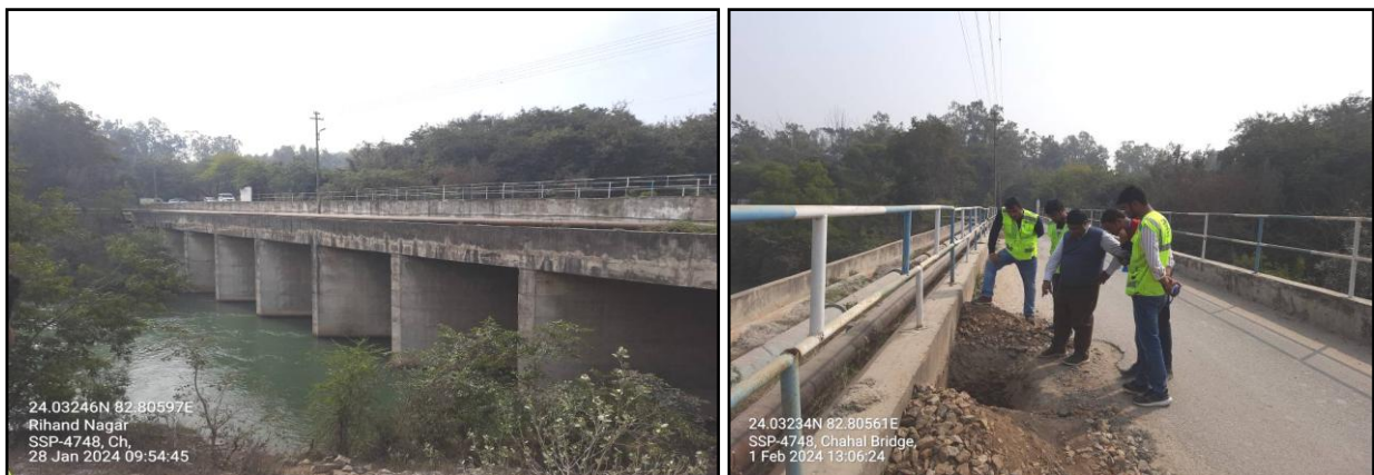
Figure 25: Typical Side View of the Chahal Bridge at STPP of NTPC, Rihand (b) A Typical View of Inspection of Crust Thickness of Road
