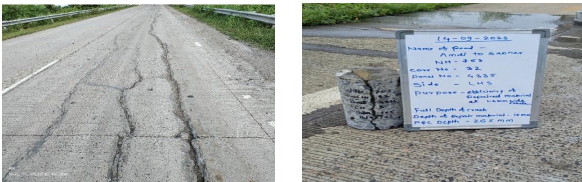
Figure 5: Investigation of distress in PQC, propagation of crack depth to PQC and DLC layer
