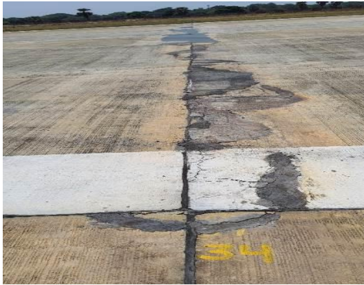
Figure 8: Deteriorated condition of the repaired expansion joint
