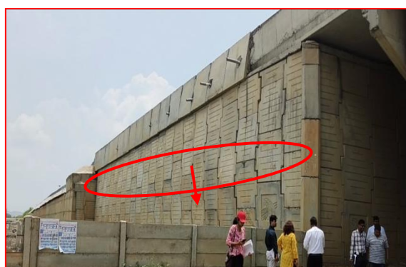
Figure 4:(b) Bulging of panels (RHS)
