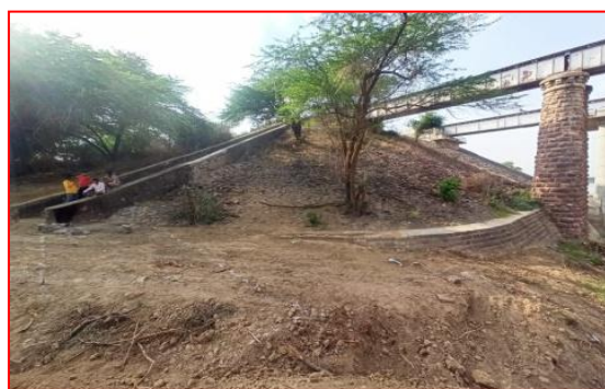
Figure 11: (d) Site Showing the Rail Embankment, RRM wall Abutment and Pier-1 towards Kota End
