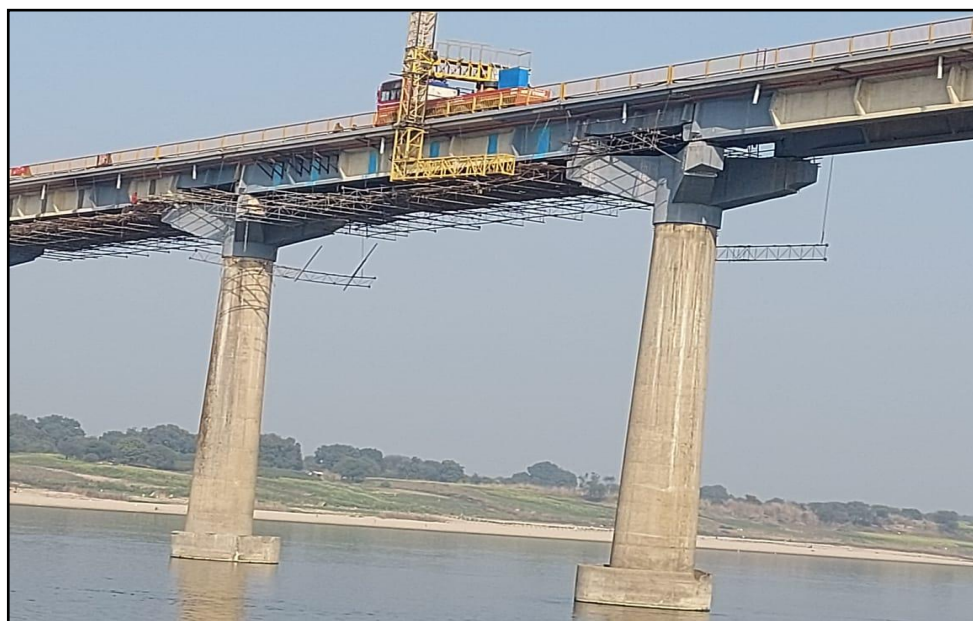
Figure 21: A View of Inspection through Mobile Bridge Inspection Unit of under Rehabilitation Yamuna Bridge at Bendaghat.
