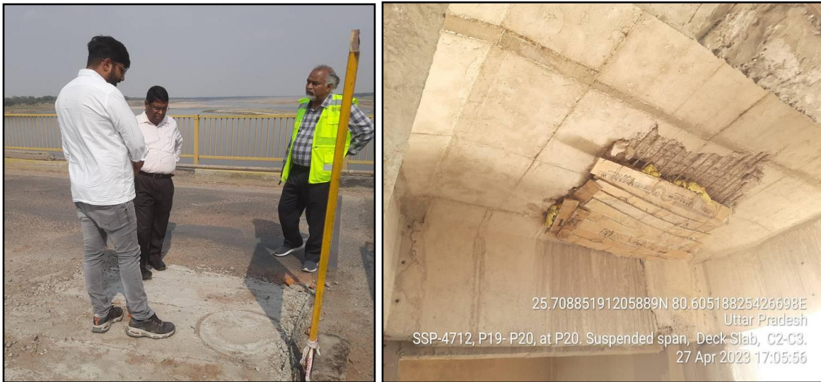
Figure 18: A View of Partially Repaired Gap Slab Span at Pier head of Pier P20 near Span P20-P21 (b) Bottom View of the Previously Partially Repaired Gap Slab at Pier Head of Pier P-20 between Cross Diaphragm C2-C3 of Yamuna Bridge at Bendaghat.
