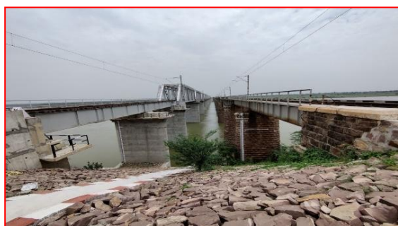
Figure 11: (a) Kali Sindh River Rail Bridge No. 34 on Kota - Beena UP rail track
