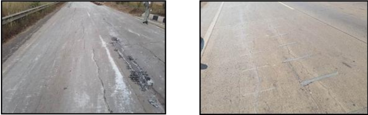
Figure 6: Typical photos showing the existing condition of the pavement at different locations
